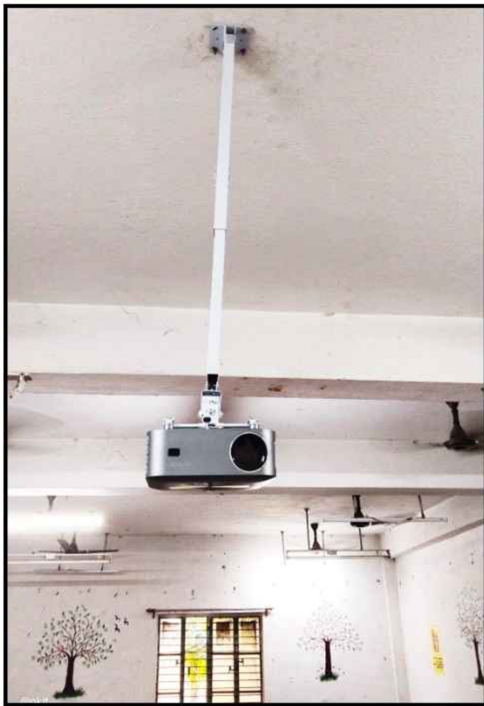
PROJECTOR INSTALLED IN ROOM NO 204
