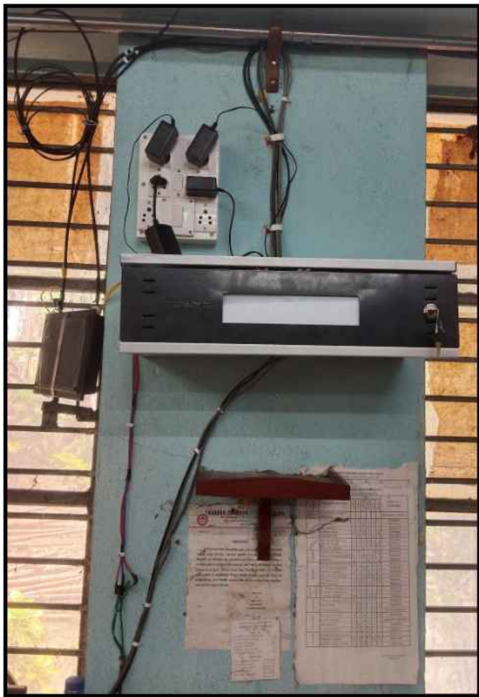
INSTALLED BOX FOR ALL NETWORKS SET UP IN OFFICE
