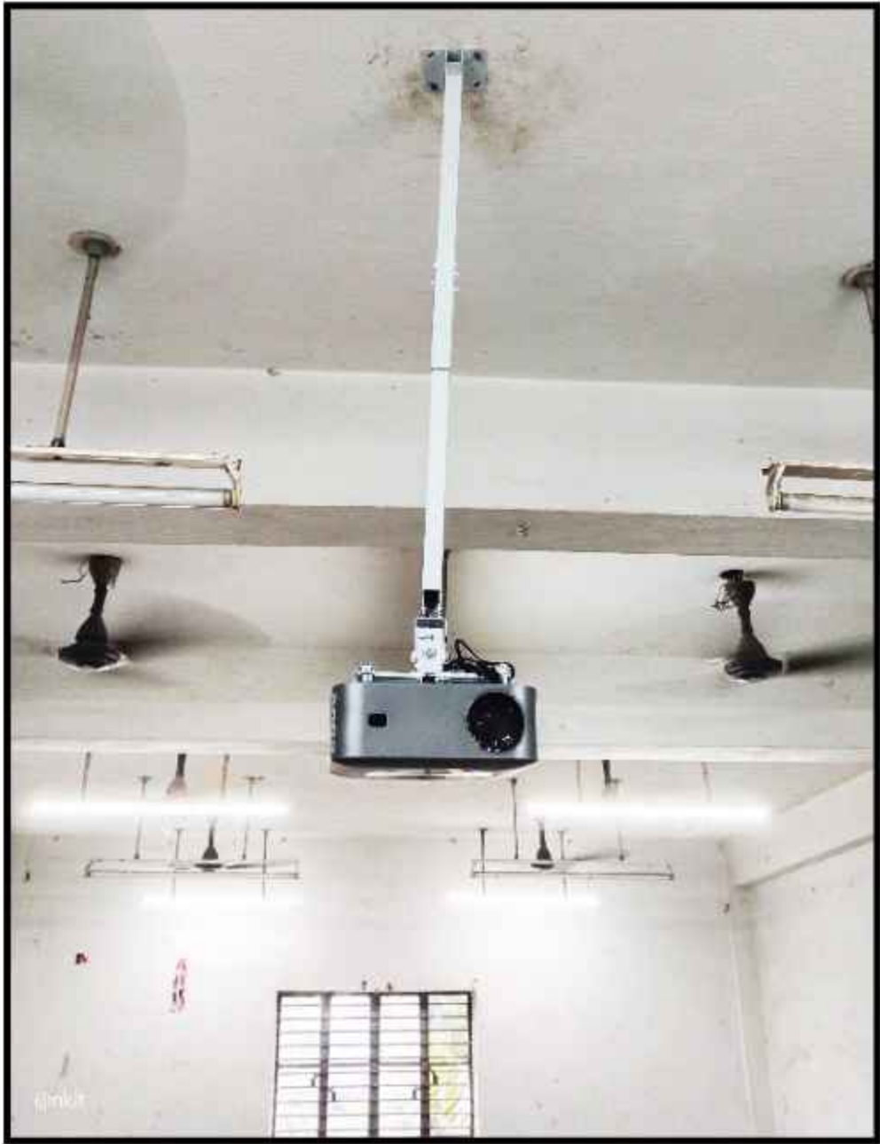
PROJECTOR INSTALLED IN ROOM NO 103
