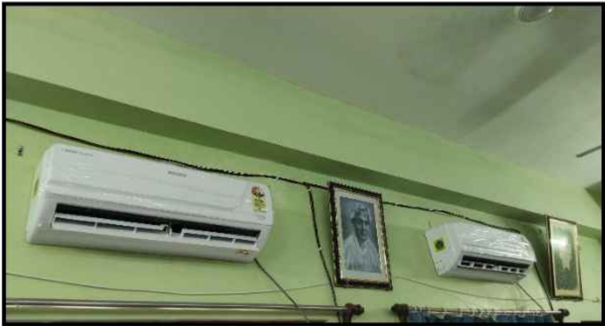
AIR CONDITIONER IN LIBRARY
