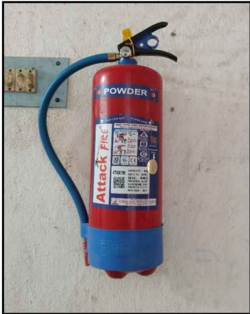
INSTALLED FIRE EXTINGUISHER IN COLLEGE BUILDING
