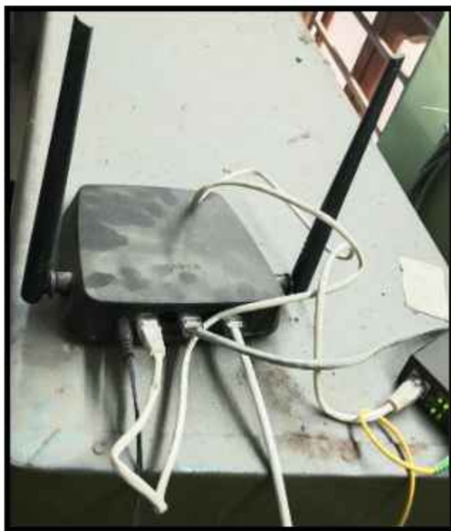
WI-FI ROUTER IN CENTRAL LIBRARY ROOM
