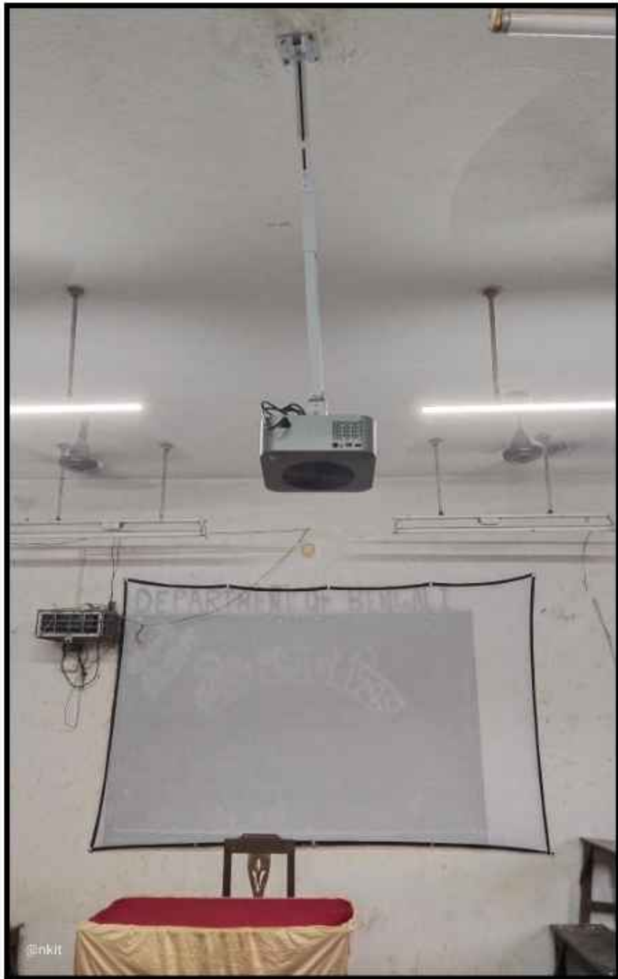
WHITE SCREEN FOR PROJECTOR INSTALLED IN ROOM NO 204
