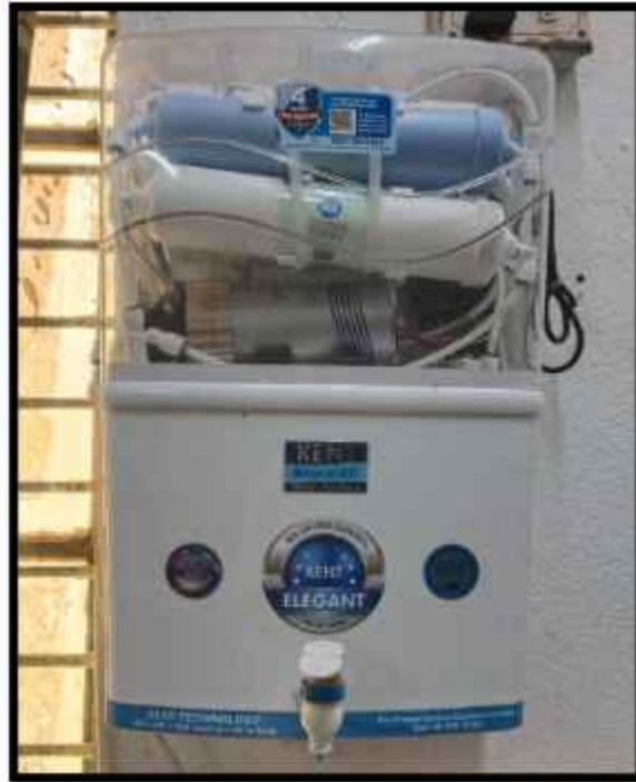
KENT RO WATER PURIFIER IN TEACHERS' ROOM
