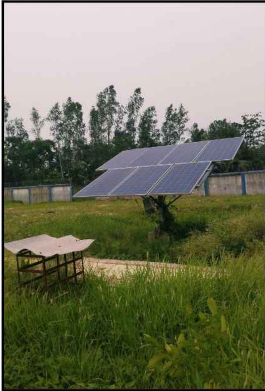
SOLAR PANEL/POWER PANEL
