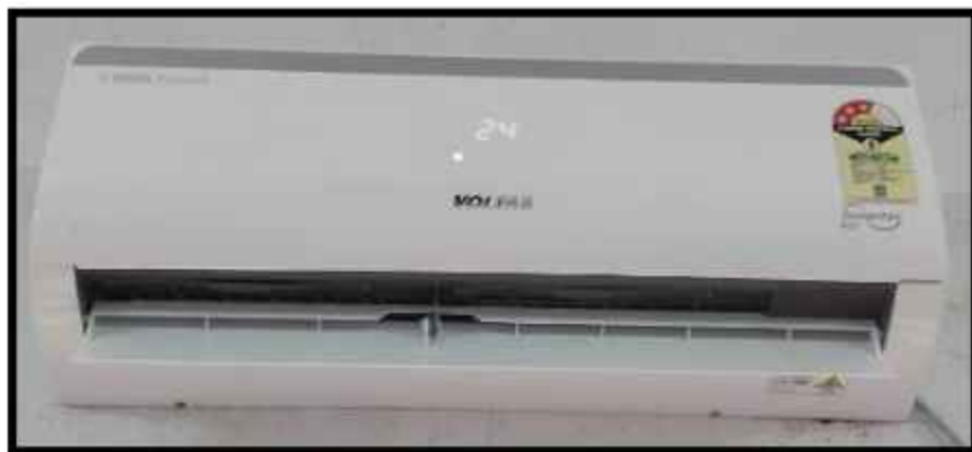
AIR CONDITIONER IN NAAC/IQAC ROOM
