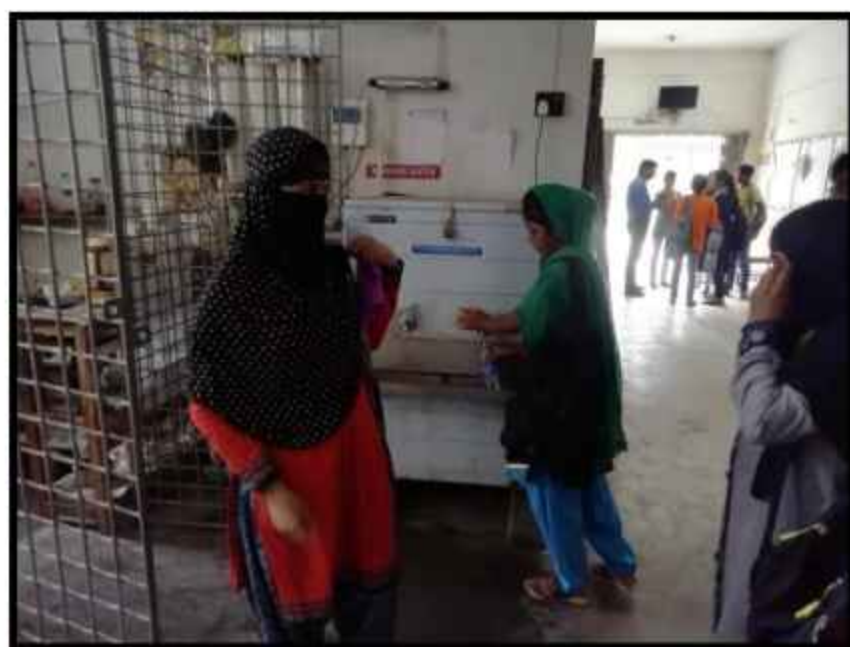
SAFE DRINKING WATER FACILITY (NORMAL AND COLD) FOR STUDENTS
